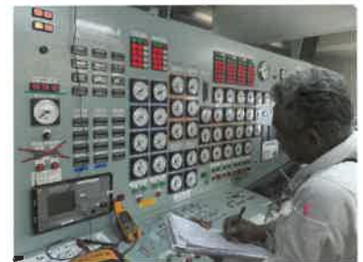
Periodic inspection of instrumentation device
